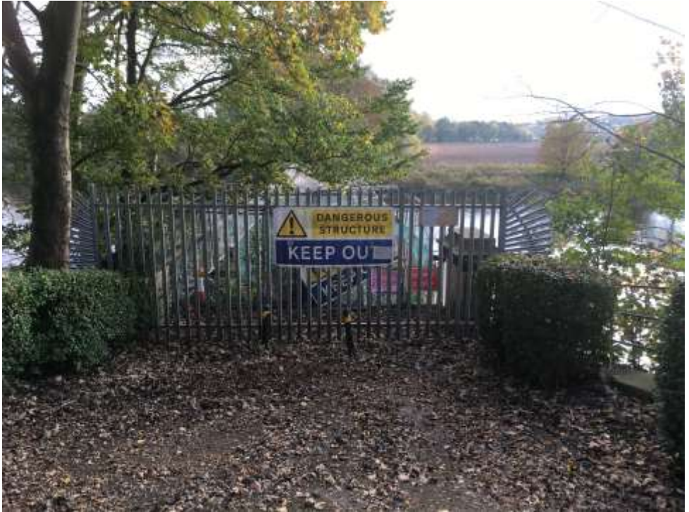
Old Tram Bridge carrying the tramroad linking the two sections of the Lancaster Canal across the River Ribble in Preston: photo supplied by IWA
